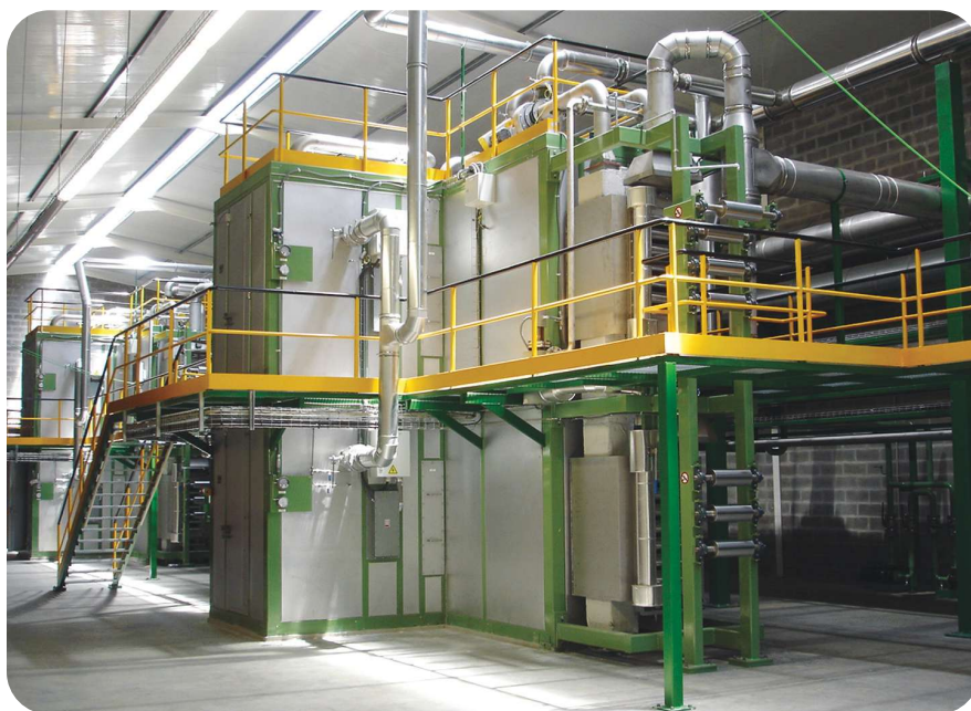
Designing the most effective thermal processing solution for production scale applications must include early consideration for energy efficiency, product quality, and throughput.
